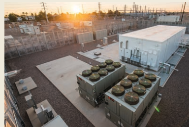
Commercial Telecom Business Unit Manager at Salt River Project Clint Poole (top) averts data center inefficiencies with his invention of SRP DataStations (bottom).
